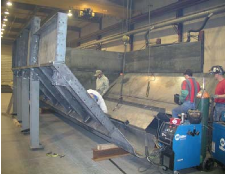
Pictured above is the SMF crew working on the rounded bottom of the carcass hopper for Swift Company in Marshalltown, Iowa.
