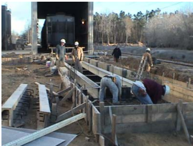
Pictured above shows Todd & Sargent crews forming the new 900 TPH rail receiving pit work.
