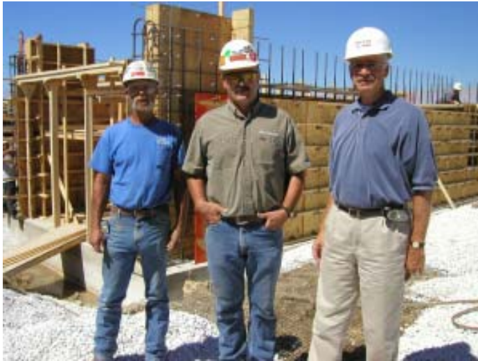
Pictured in front of the bucket elevator boot pit currently being constructed in Fort Dodge is General Foreman Dale Mittlieder, Superintendent Dennis Taggart and Fagen On-Site Project Manager Dennis Lessard.
