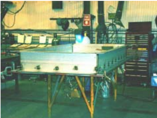
Robin Frazier welding headed anchors to a stainless steel door embed for the USDA project in Ames,
