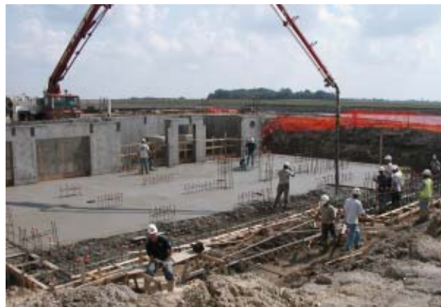
Todd & Sargent crews are working on pouring the slab for the receiving area of the Bean Storage Elevator at Harvest States in Fairmont, Minnesota.
