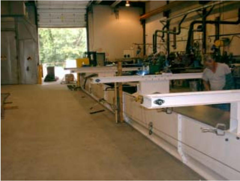
Danny Wall is pictured installing conveyor lids on the truck/rail loadout conveyor for Buhler, Inc.
