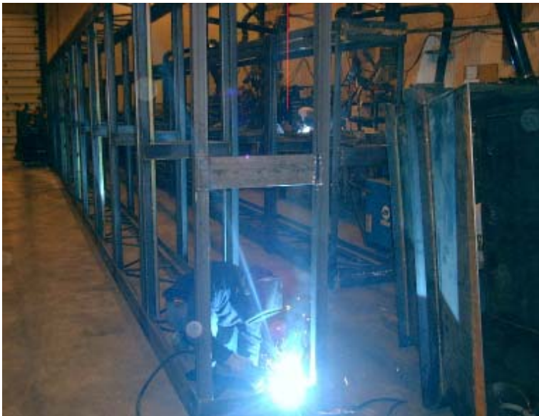
James Stofer is doing some final welding on one of many unit sections for Ball Plastics, Delran, New Jersey plant.
