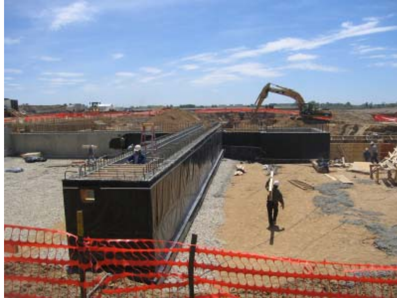
Picture above shows construction of the tunnels, forming for the tunnel roofs, waterproofing and backfilling at the Charles City, Iowa facility.
