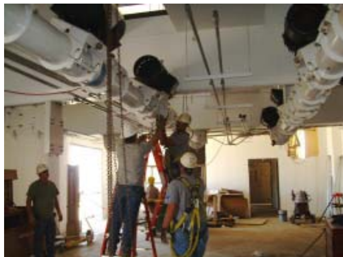
Todd & Sargent's Jesse Perez and Ryan Zuck along with SCA employees John Patchett and Roger Phillips are installing the roll stand motor mounts at the Hopkinsville facility.
