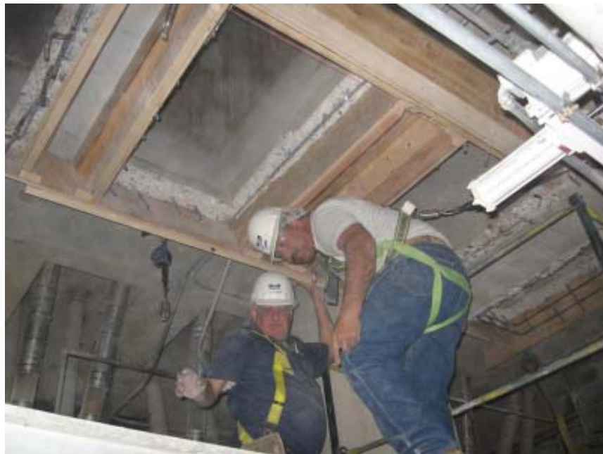
Todd & Sargent Leadmen Steve Johnson and Juan Manual Lopez are in the process of installing equipment at the Horizon Milling facility.
