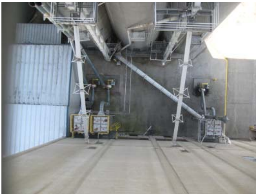
Pictured above is the area where the new milling expansion will be located at the Iams Company - Procter & Gamble Pet Care facility in Leipsic, Ohio.
