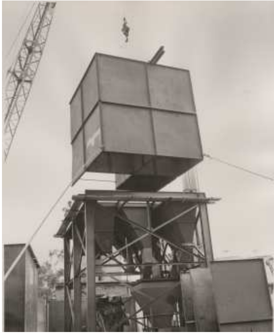
Typical Todd & Sargent Steel Bins
