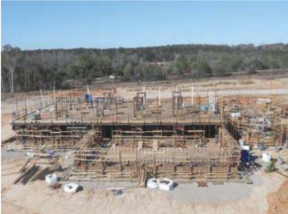
Photo shows Wayne Farms feedmill ready to slip on January 18, 2016. Pelleting core is in front, dual truck loadout bays at left, and mill batching and ingredient tower in center.
